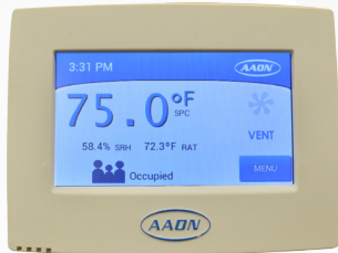
Factory Provided AAON Touchscreen Controller
