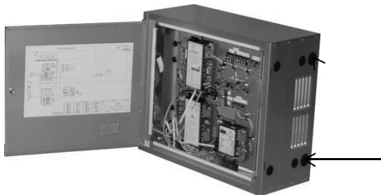
Figure 15 - External control box electrical connections
