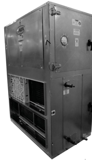
Figure 16 - V3 internal control panel electrical connections
