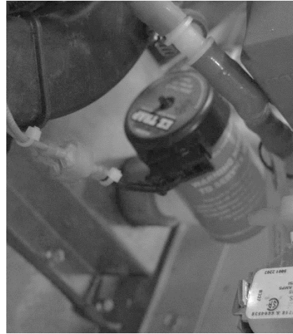
Figure 50 - Condensate Drain Overflow Switch
