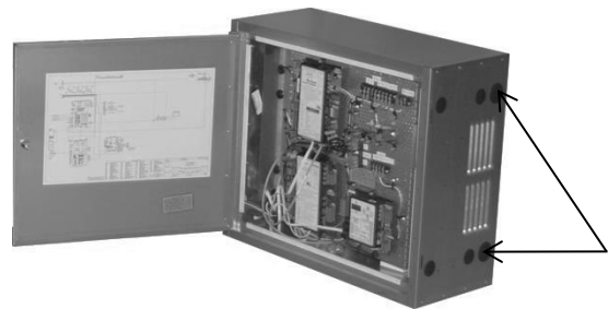
Figure 16 - External control box electrical connections
