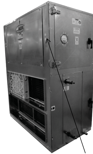
Figure 16 - V3 internal control panel electrical connections
