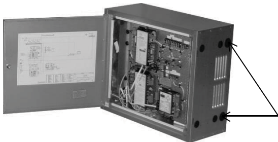
Figure 15 - External control box electrical connections
