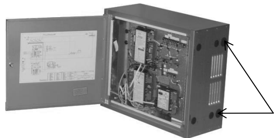
Figure 17 - External control box electrical connections
