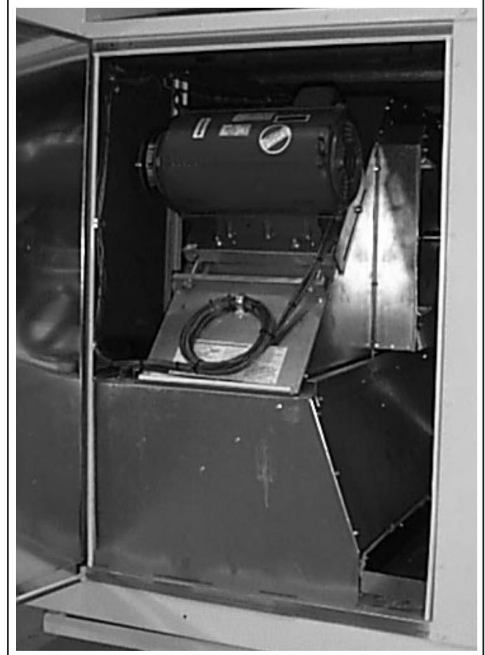
Typical slide-out blower section
