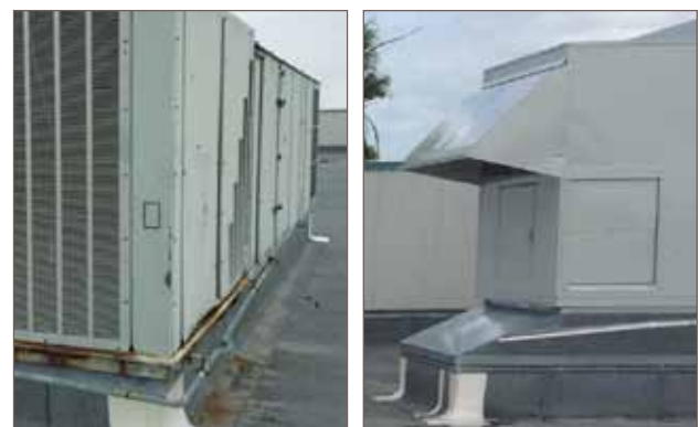
On the left is the original equipment and on the right is then new AAON equipment with corrosion resistant exterior paint.
