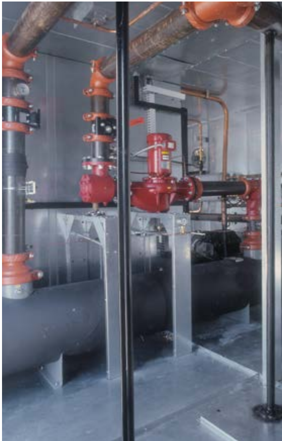
Factory Installed Chiller and Pumping Package
