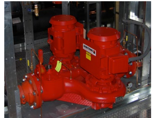
DualArm Pumping Package
